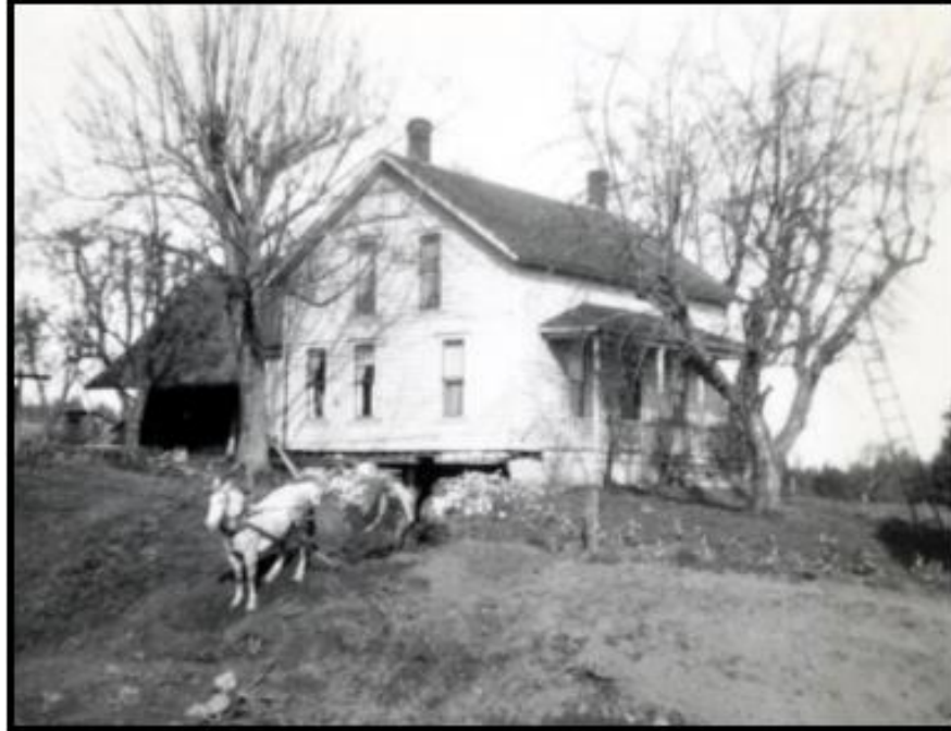
The Rebstock house as it appeared during the 1940s. Here a basement is being built under the house.
