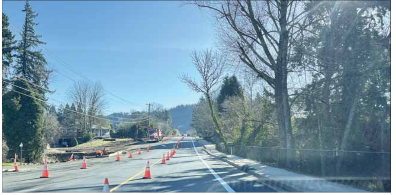
A view of King Rd. looking east shows crew members and equipment along the Superblock.
