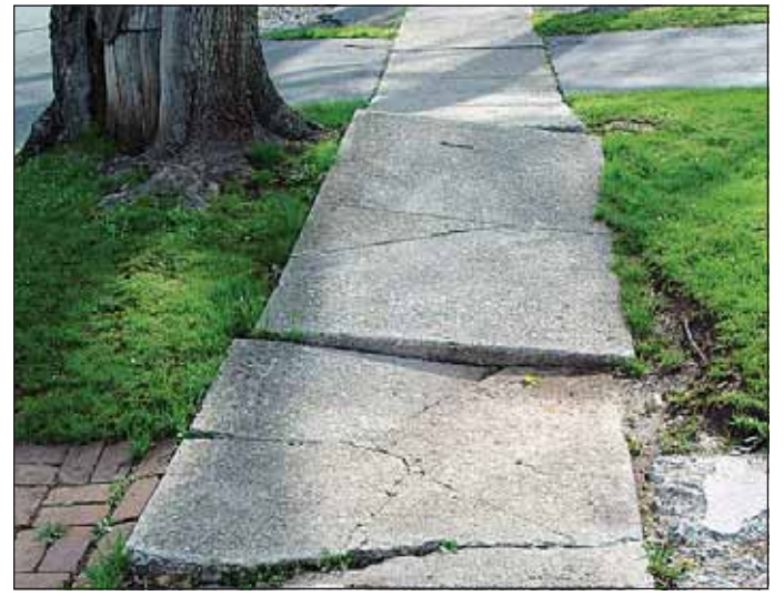
Watch out! Sidewalk concrete that has become disjointed, cracked, broken and uneven is a hazard. In Happy Valley, property owners are responsible for ensuring sidewalks adjacent to their homes and businesses remain in good working condition.
