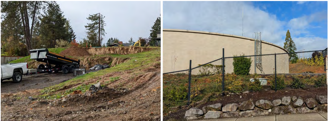
Figure 4-3. Construction (left) and Water Storage Facility (right) in Happy Valley residential areas
