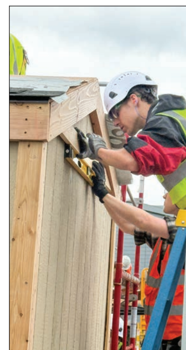
A student from the advanced construction class of Sabin Schellenberg Professional Technical Center looks over the rough plans of a shed they built for the Construction Industry Education Foundation Design Build Competition.
