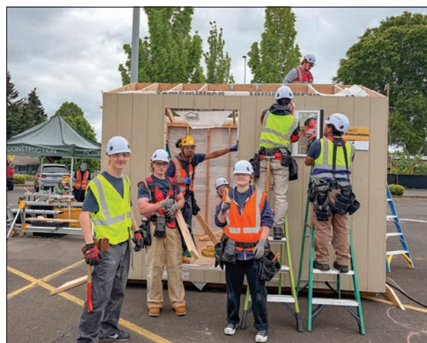
A student from the advanced construction class of Sabin Schellenberg Professional Technical Center works on the side of a shed they built for the Construction Industry Education Foundation Design Build Competition.
